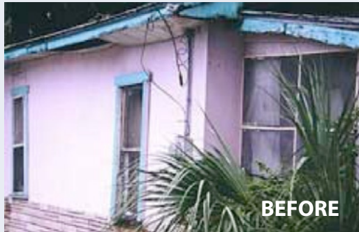
Abandoned building. Source: ATSDR Case Study, 2017.
