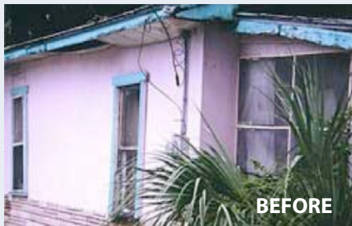
Abandoned building. ATSDR Case Study, 2017
