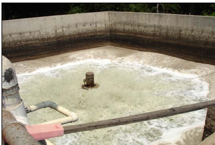
Treated wastewater prior to being spray applied to crop fields. Because of constant aeration, the original odors have been greatly reduced.
