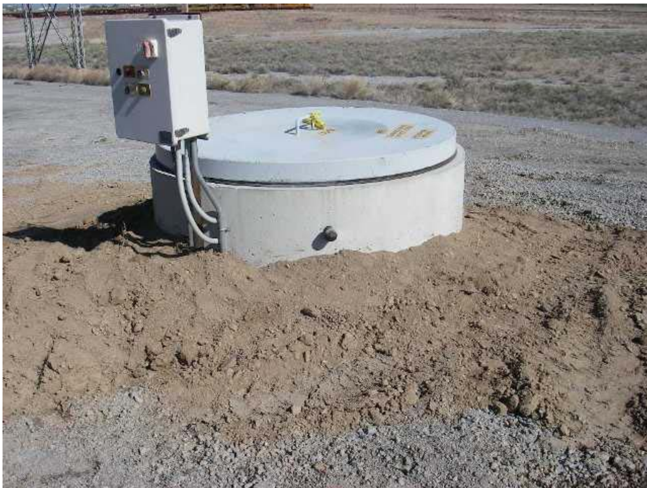
Pond 15S lift station 1 (LS1) after improvements to prevent gas seepage. This is the location of the phosphine ambient air samples that prompted the initial letter health consultation in June.
