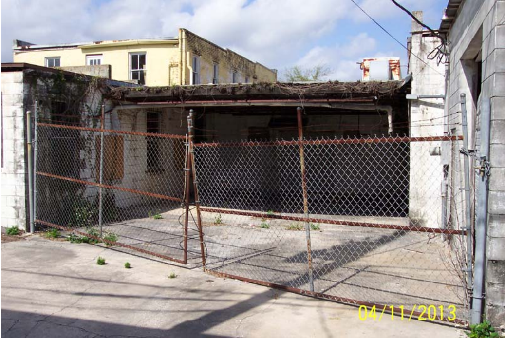
Photograph 3. East side of SDC site, view of locked gate at rear of building looking NW.
