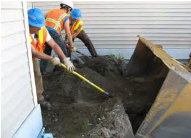
Figure 7. Contractors shovel petroleum, oil, and lubricant (POL) contaminated soil into a loader for transport to a soil cell.
