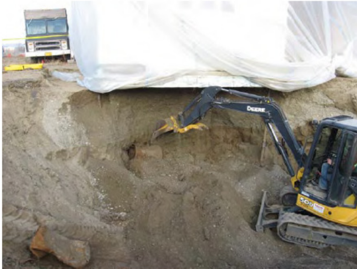
Figure 5. Exposed drums under foundation during trial excavation
