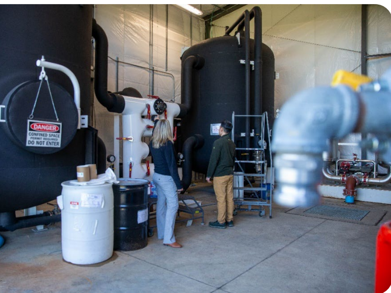
Figure 2. The groundwater treatment system building at NASA's Wallops Flight Facility in Virginia. NASA/Patrick Black
