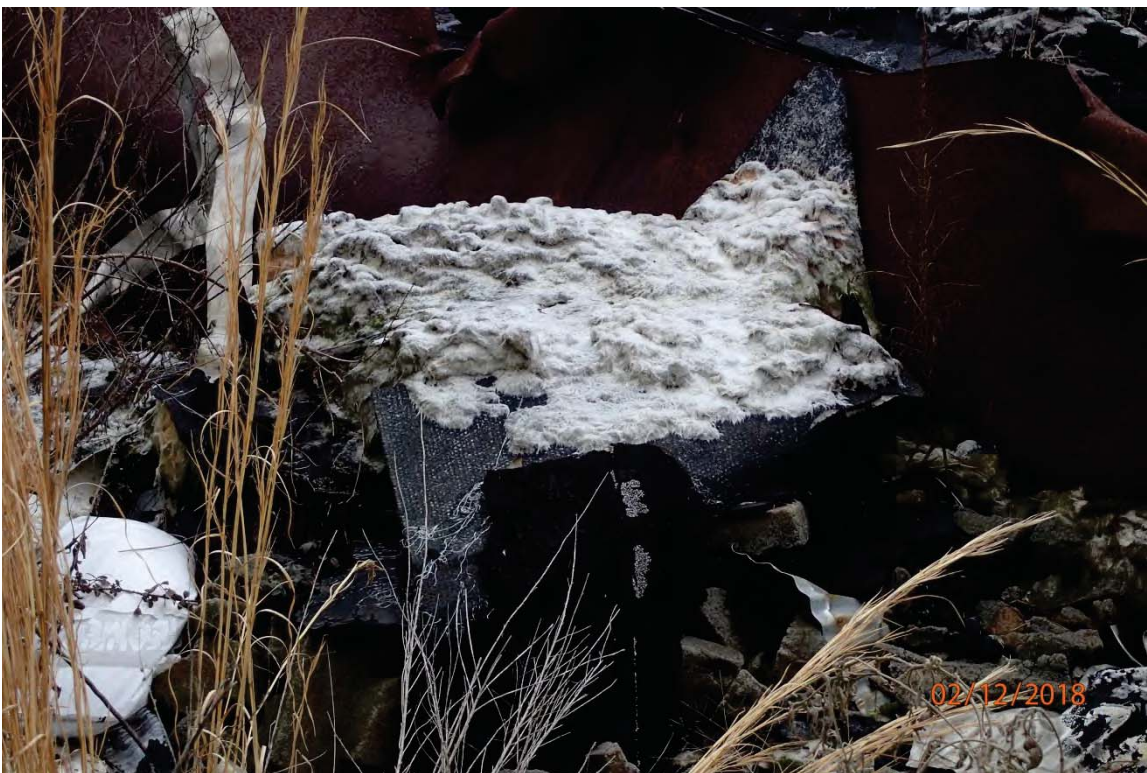
Photo 24: Close up of suspected asbestos insulation material at former asphalt tank near Industrial Area. 2018
