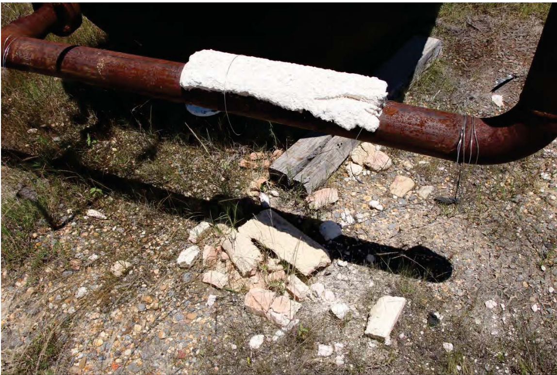
Photo 22: Suspected asbestos insulation from pipe exposed and on ground at Industrial Area. 2016
