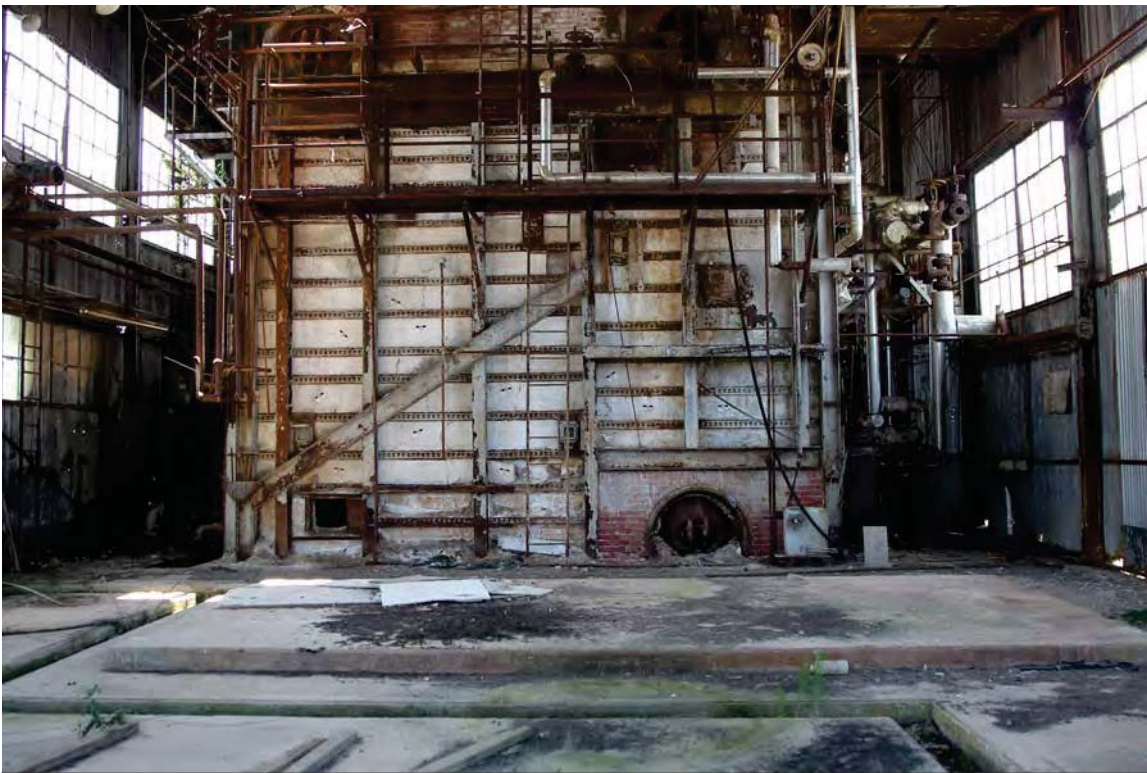
Photo 26: Block asbestos insulation at boiler house near Industrial Area (Asbestos danger signs posted on building). 2016
