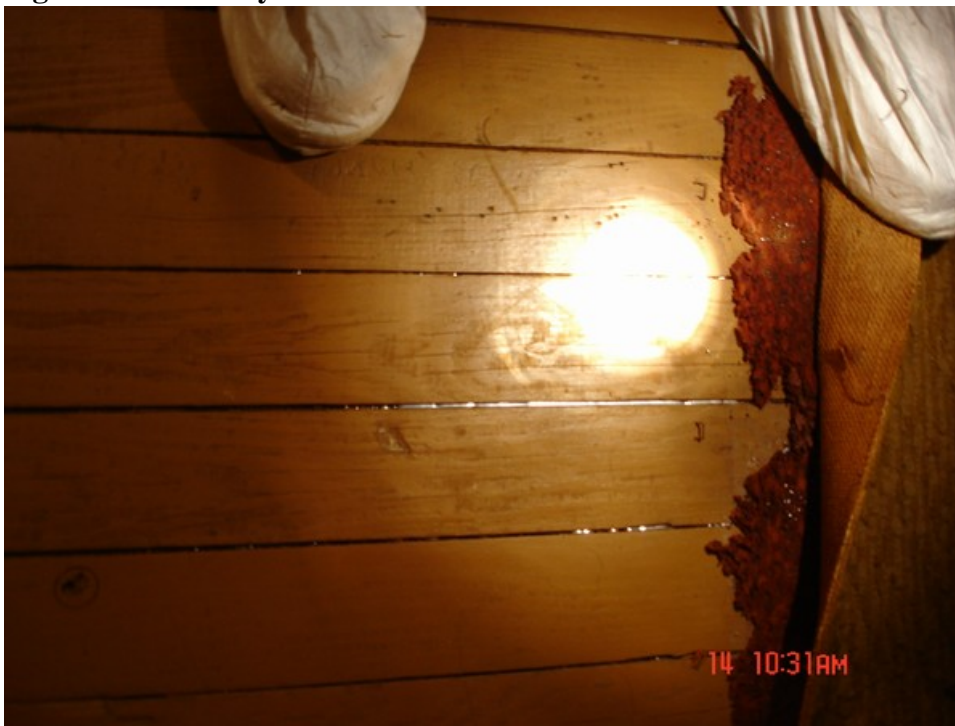
Figure 1a: Mercury Contamination in Floorboards of a Residential Home.
